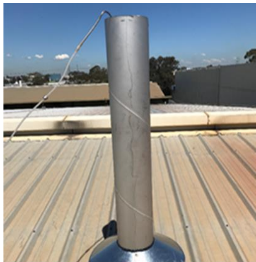
Figure 3 – Hot Oil Heater Stack
